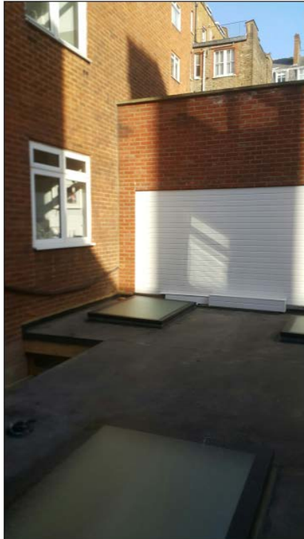
South (rear) elevation with newly erected lower ground floor extension in foreground
